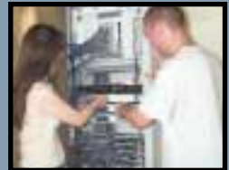
Networking – Second year Networking students examine cabling and networking devices in a communications cabinet.
